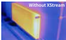
Radiator with trapped air at the top and dirt blockages at bottom
