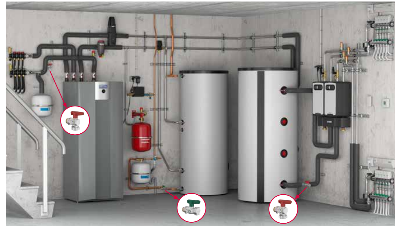
Example: small boiler room
