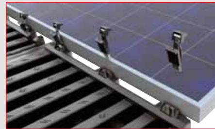
Secure the PV panels with clips and pass the cables through the ducts
